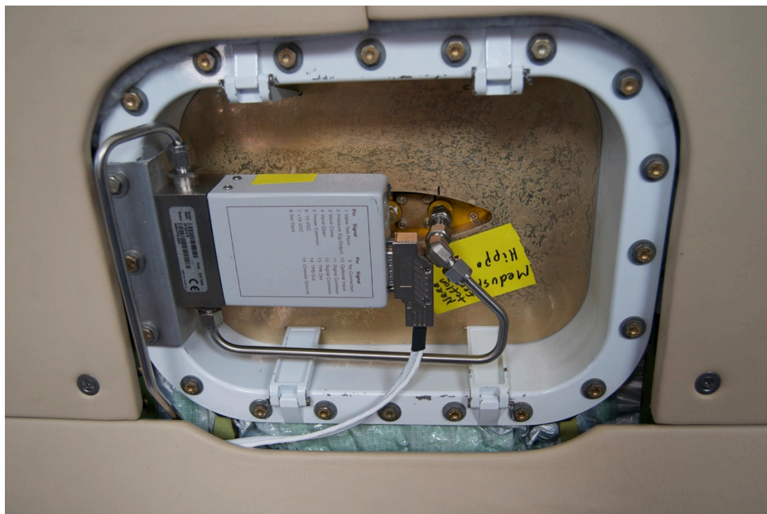
Figure 2.8. “Lasagna pan” at the bottom of the MEDUSA HIMIL, as seen by the sampler’s operator from the cabin. Air passes from the HIMIL inlet along electropolished ¼” stainless steel tubing to pass-through bulkhead fittings on the right, and to the upstream pressure controller (PC). All sample air downstream of the PC is kept at a constant pressure, which is determined by one of 2 flow regimes (high flow/low alt; low flow/high alt).
